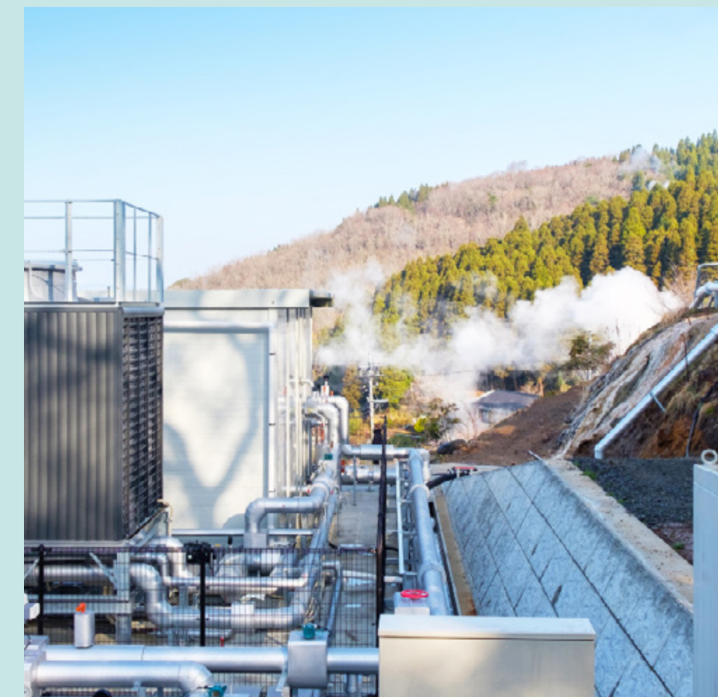
The Sansui geothermal power plant in Japan. Photo: Baseload Capital.
