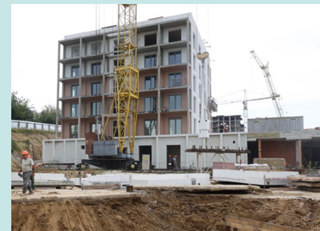
The first new urgent housing building under construction in Lviv, Ukraine. Photo: Lviv City Council.
