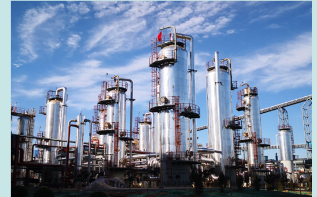
The Shunli plant in China is the world's first commercial CO 2 -to-methanol plant. Photo: Carbon Recycling International.
